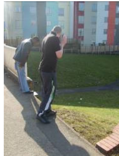
Lack of barrier on bridge on Park Grange Road
